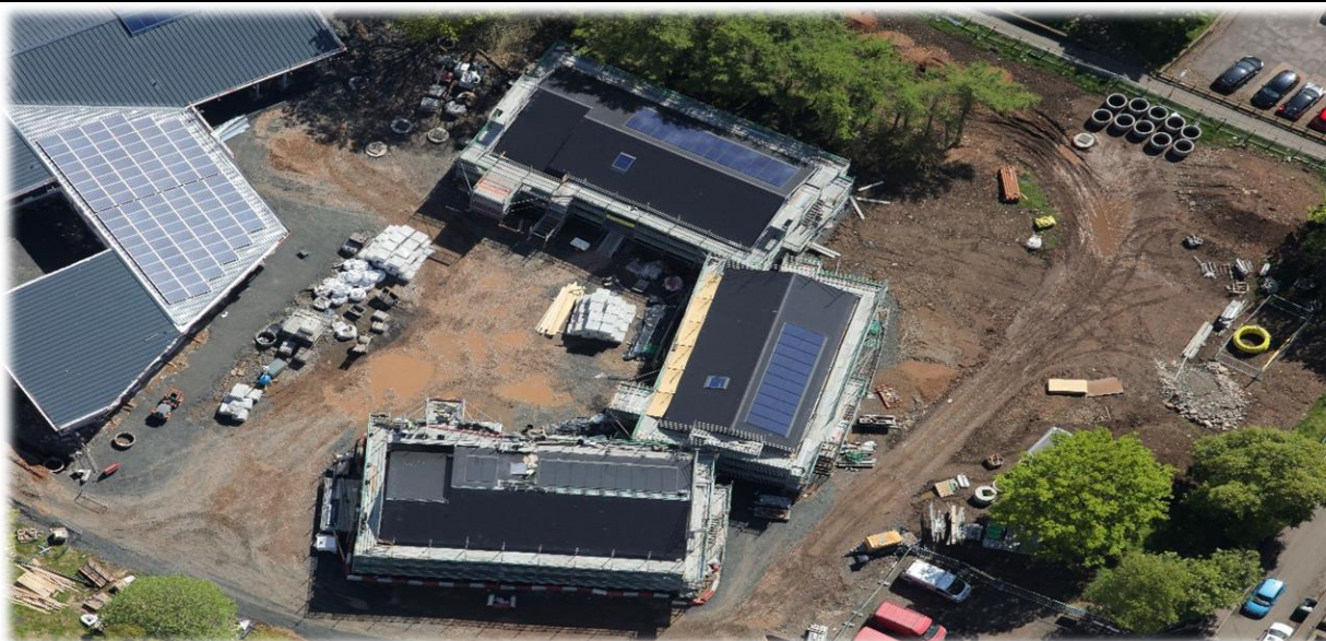
CCU, Dundee, May 2021. Note use of Photovoltaic / solar panels on the Hub Building and house-roofs
